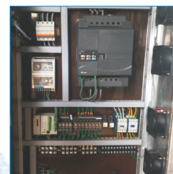
Main Electrical Panel
