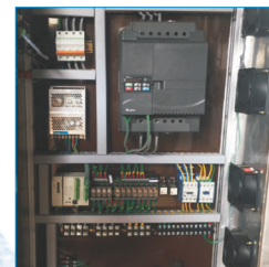
Main Electrical Panel
